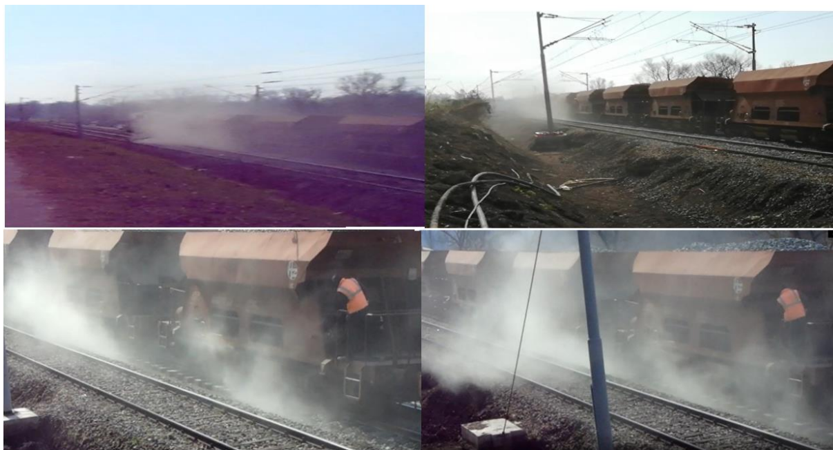
Figure 8. – Recordings of railway works of unloading the crushed stone on March 08, 2021 (image source: AIN)
