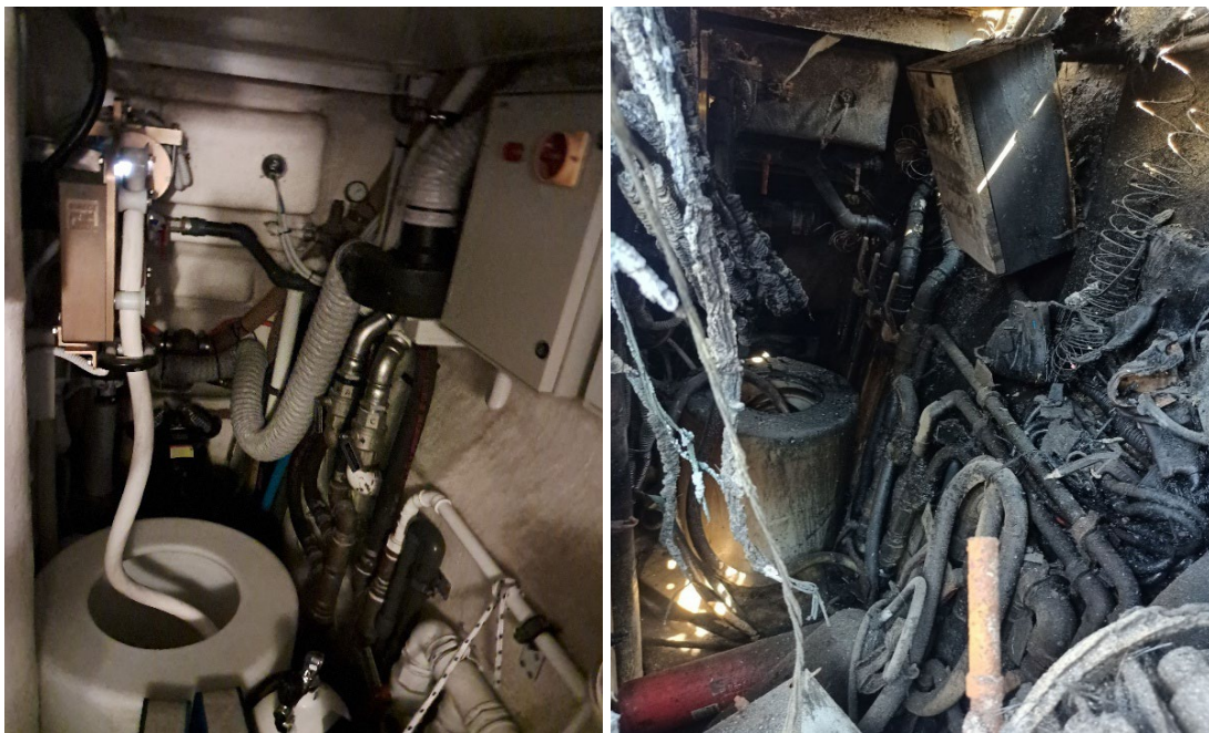
Figure 5. Technical area – aft section, on the sister yacht and on the burned yacht (source: AIA 1 )
